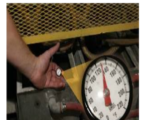
Image 29 – Water tank temperature reading
